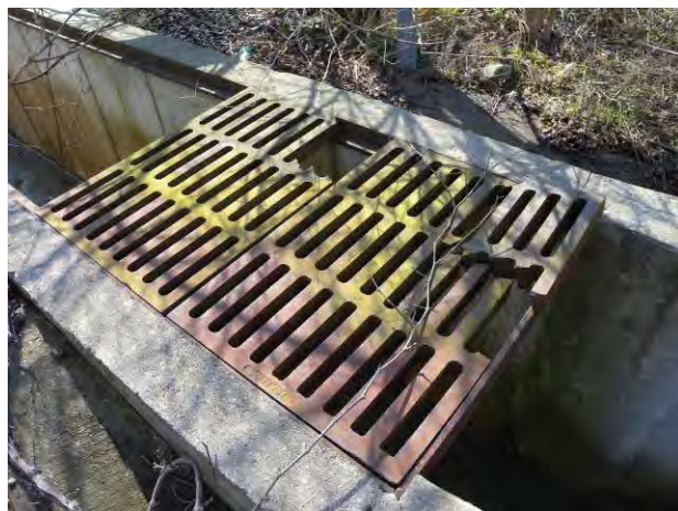
Figure 20. Single Remaining Grate
