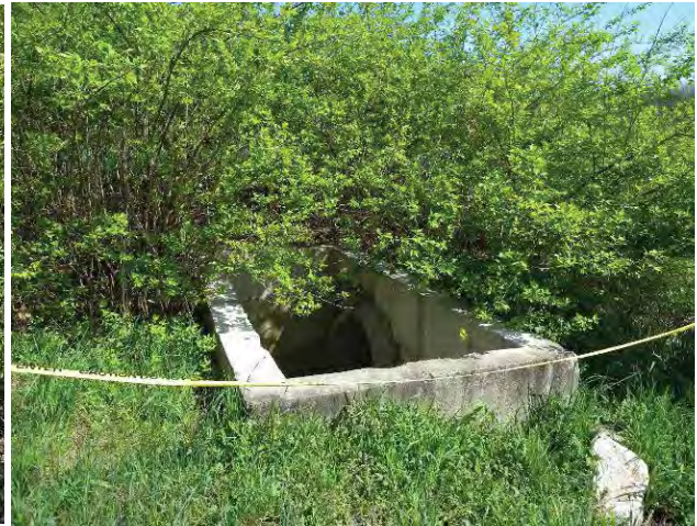
Figure 12. Storm Drain from Which Grate Was Stolen in Parcel 8
