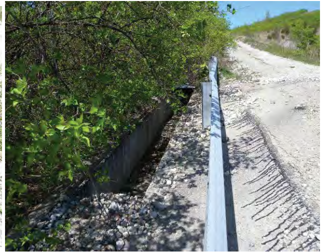
Figure 10. Section of Parcel 8's Western Site Boundary from Which Grates Were Stolen, Looking North and Uphill
