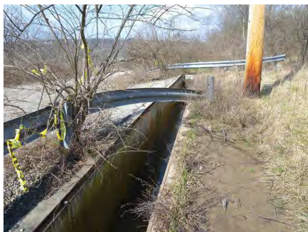
Figure 22. Section of Storm Drain from Which Grates Were Stolen
