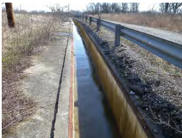
Figure 23. Section of Storm Drain from Which Grates Were Stolen, Looking East
