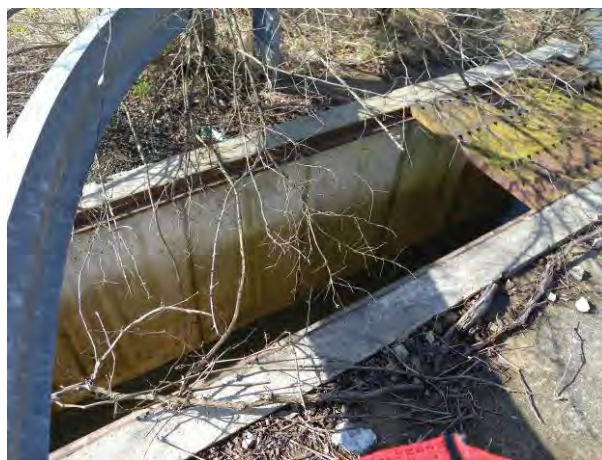
Figure 21. Single Remaining Grate
