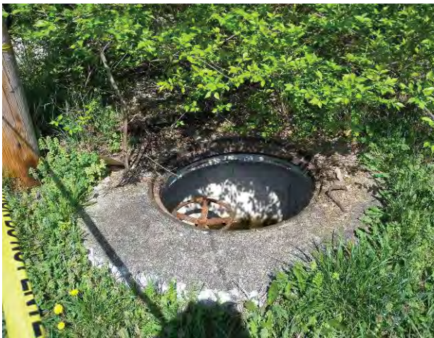
Figure 13. Manhole from Which Grate Was Stolen in Parcel 8
