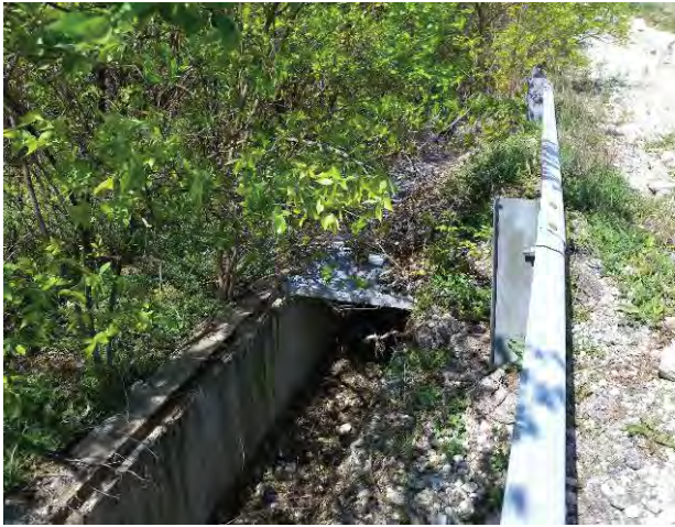
Figure 9. Storm Drain from Which a Grate Was Stolen in Parcel 8, Looking North and Uphill Along the Western Site Boundary
