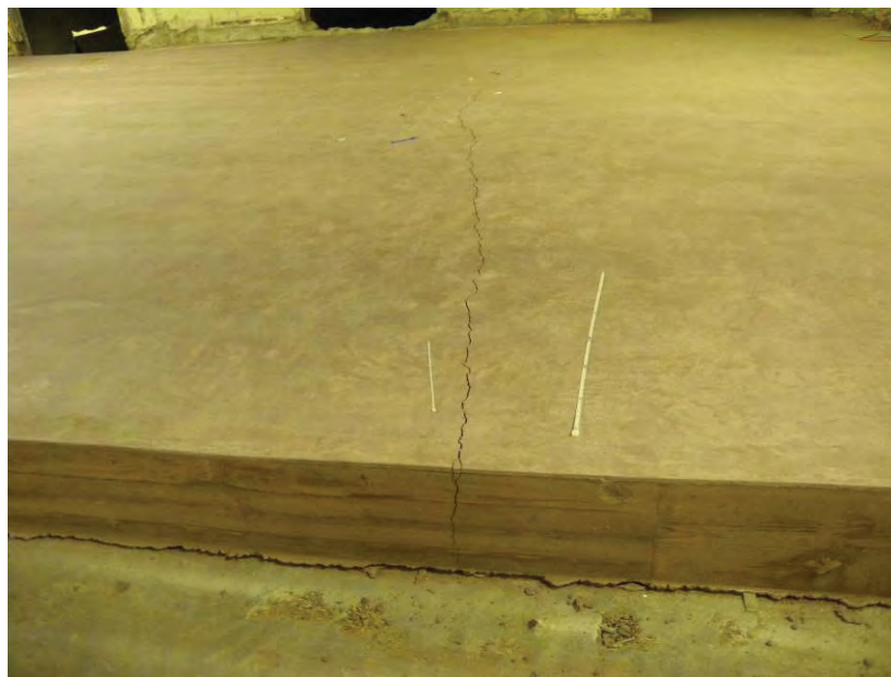
Figure 14. 2012 Photo of Crack in Red Concrete Slab in T Building Areas Where Penetration of Concrete Floor is Prohibited Without Prior Approval
