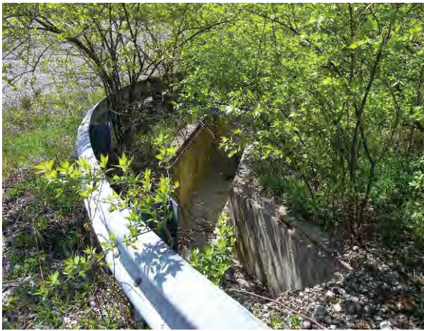
Figure 11. Storm Drain from Which Grates Were Stolen, Looking Southwest in Parcel 8
