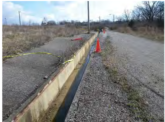
Figure 25. Section of Storm Drain from Which Grates Were Stolen, Looking East from Center Roadway
