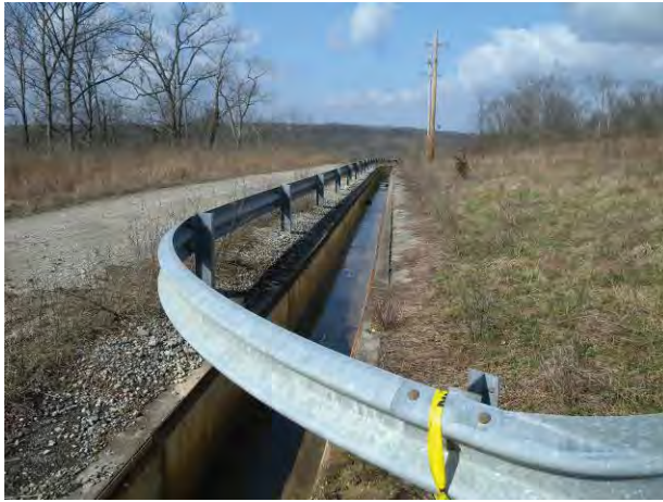
Figure 24. Section of Storm Drain from Which Grates Were Stolen, Looking West from Center Roadway
