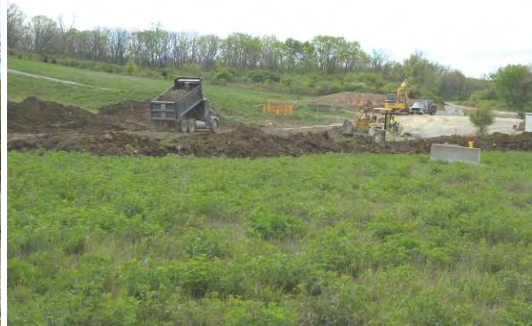
Figure 17. Work on Spine Road in OU-1 Area, Looking Southeast from Roadway. Well P053 is in Center Right of Photo.
