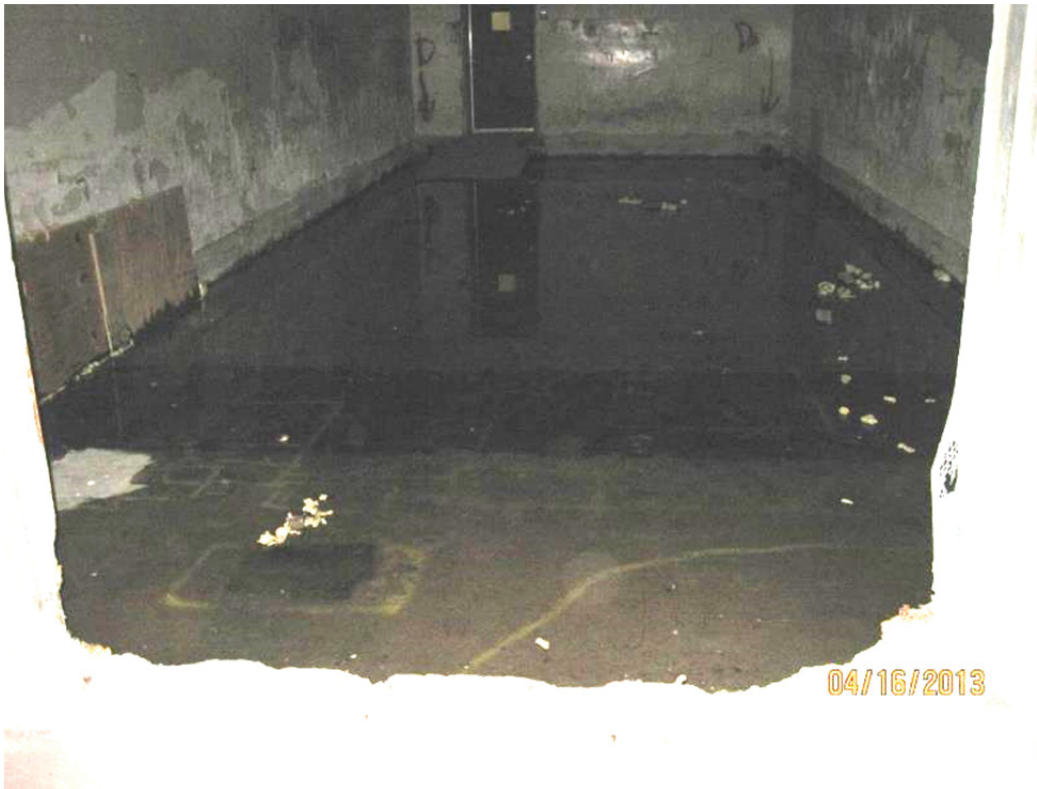
Figure 20. Standing Water Caused by Sump Pump Failure in T Building Room 58, Observed During the IC Walkdown
