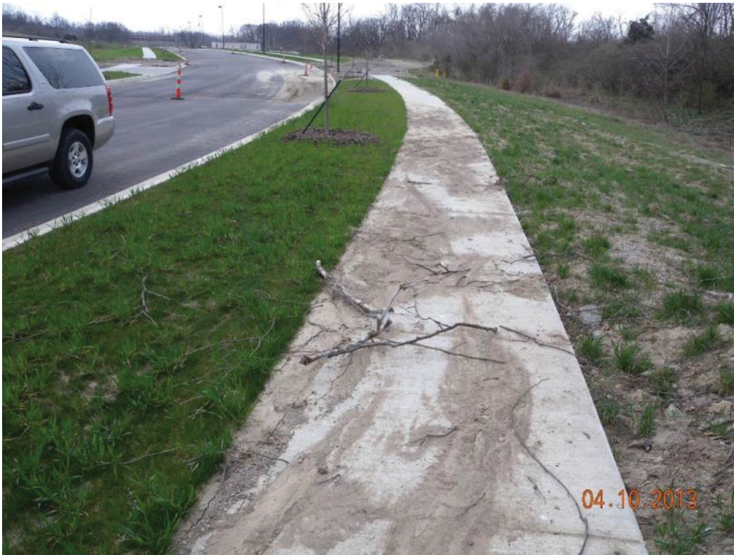
Figure 10. Erosion Problems North of Former Outfall 002
