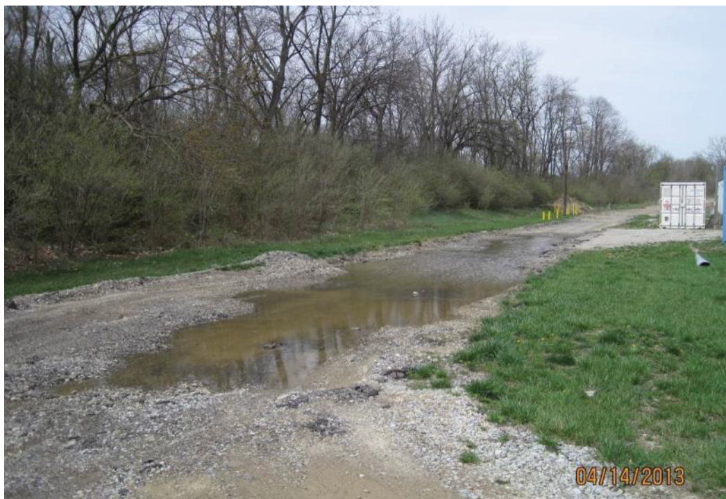
Figure 13. Drainage Issues in Roadbed Southwest of OU-1 Pump and Treatment Building 300 and Trailers 1 and 16
