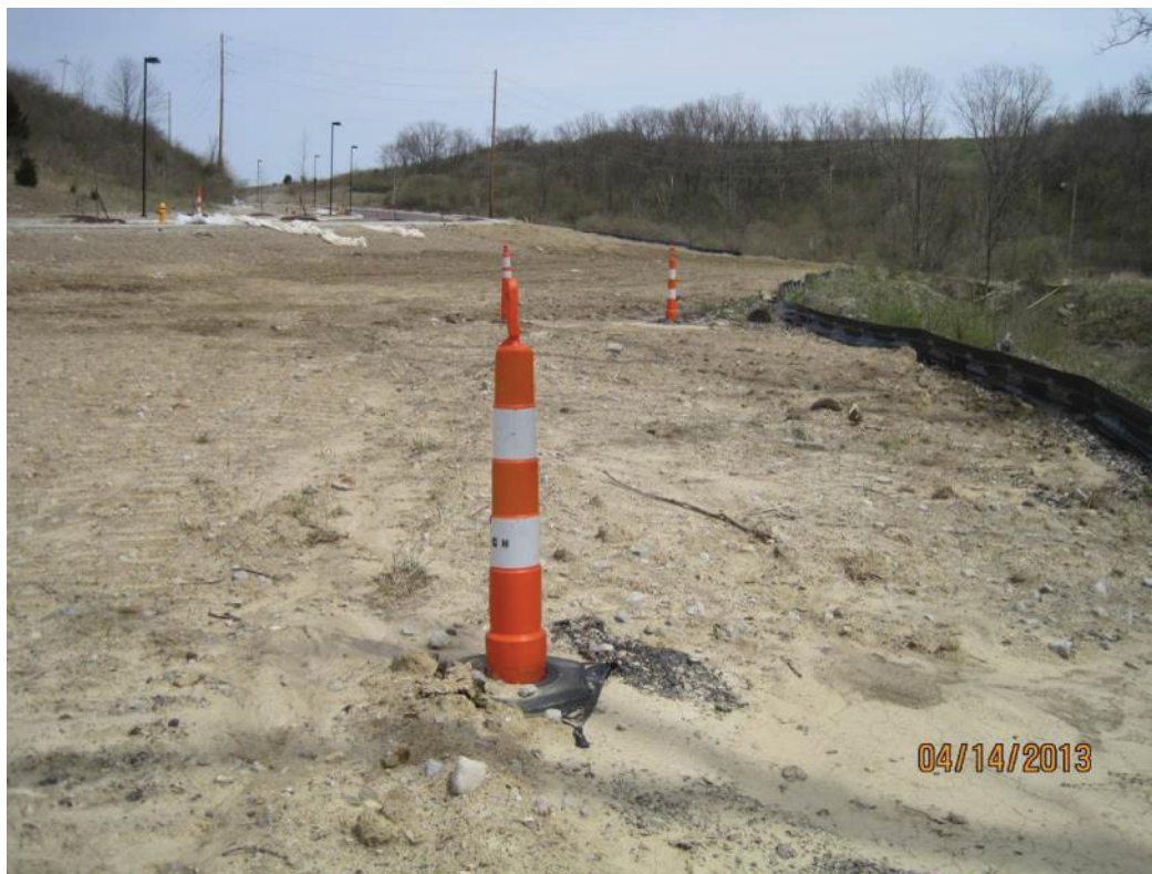
Figure 9. Erosion Problems South of Vanguard Blvd. near Well 0346
