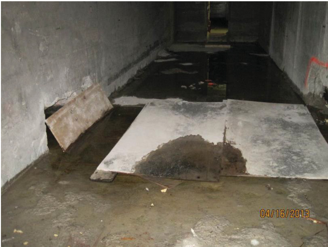
Figure 18. Standing Water Caused by Sump Pump Failure in T Building Room 57, Observed During the IC Walkdown
