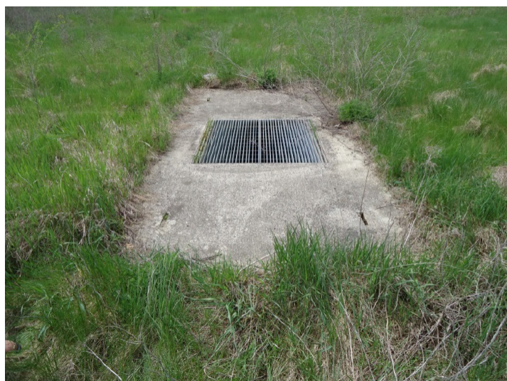
Figure 11. Catch Basin (7 ft × 14 ft)
