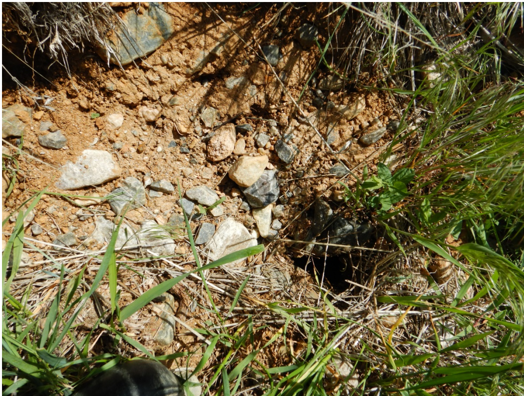
Figure 7. One of Five 1–2 Inch Holes Found Along the East End of the Previously Reported Scarp Above East Berm 4
