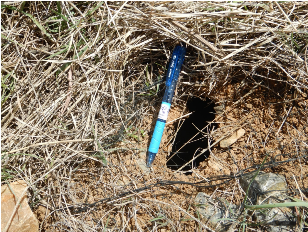
Figure 7: A 2-inch by 3-inch hole in the west-central section of the berm 5 channel
