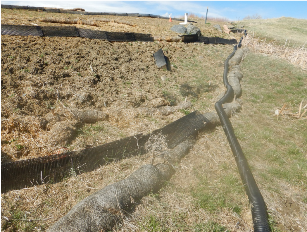
Figure 2: Looking northeast to the toe of the regraded 2017 slump area blocking the lower segment of the EPC
