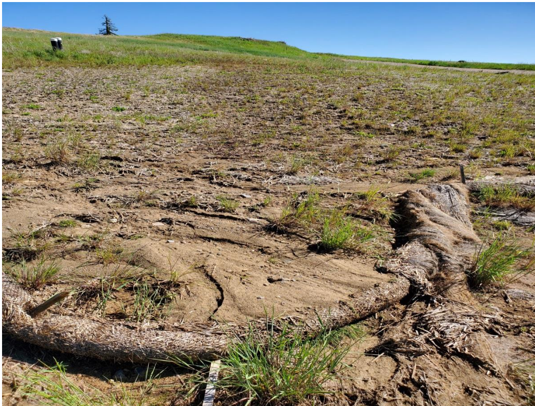
Figure 3. Looking Northeast at the Rills and Sediment Buildup on East Supporting Hillside
