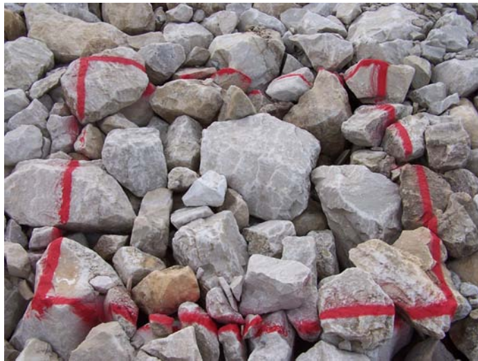
Photo 12. Cell side slope rock test plot TP2; bottom of north side slope (2005 Inspection).
