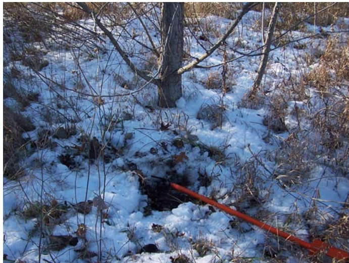
Photo 9. Manhole No. 3 on the NPDES discharge pipe. Note tree next to the manhole.
