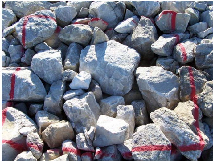
Photo 13. Cell cover rock test plot TP2; bottom of north side slope (2006 Inspection).
