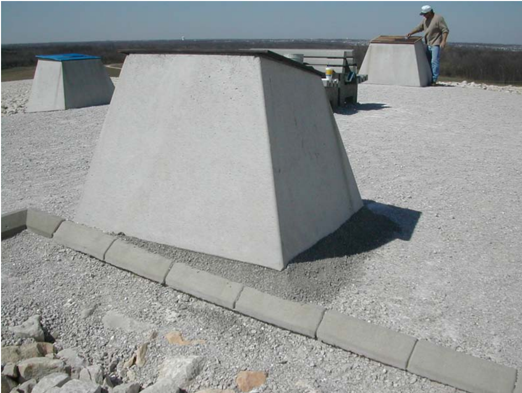
Photo 8: Repair of the erosion under the corner of the pedestal on top of the disposal cell.
