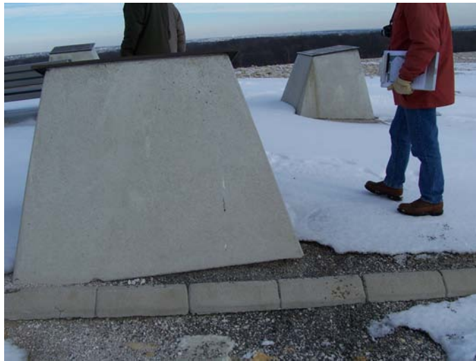
Photo 23. Corner of Pedestal on the SE Corner. Shows erosion under the bottom that had been repaired last year, but is reoccurring.
