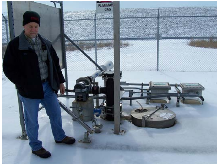
Photo 20. LCRS sump manhole.
