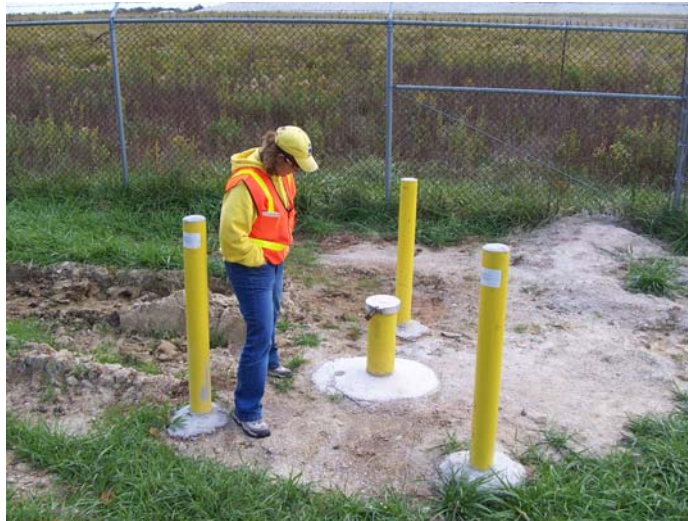
Photo 2. Recently installed monitoring well MW-4042 on the Army property.
