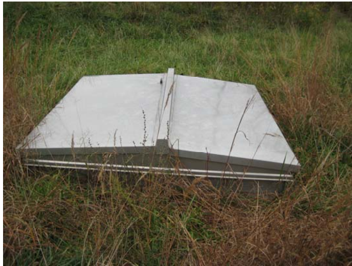
Photo 4. Water vault on MDOC property (unlocked).
