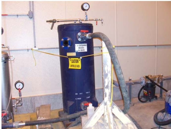
Photo 26. Ion Exchange vessel.
