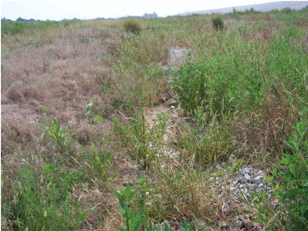
Photo 7: View upslope of repaired gully near Area #3 and newer rill forming to the left of the repair; note stabilizing vegetation in newer rill.
