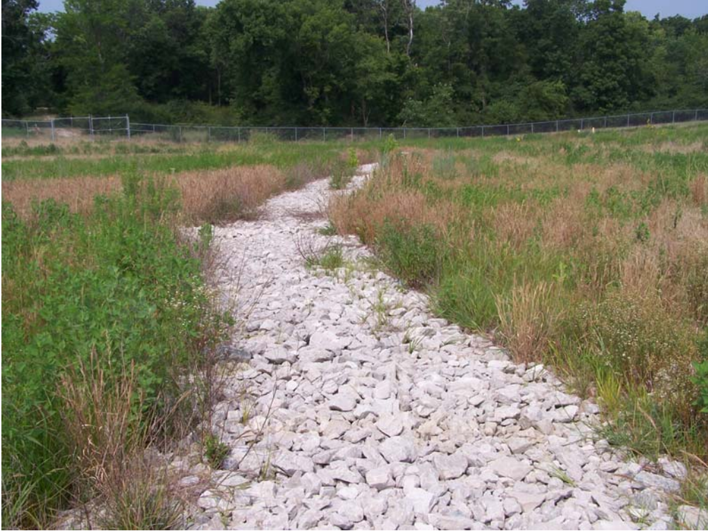
Photo 4: View downslope of repaired gully near Area #3; note vegetation encroaching on edges of repair. This repair is effectively controlling erosion.
