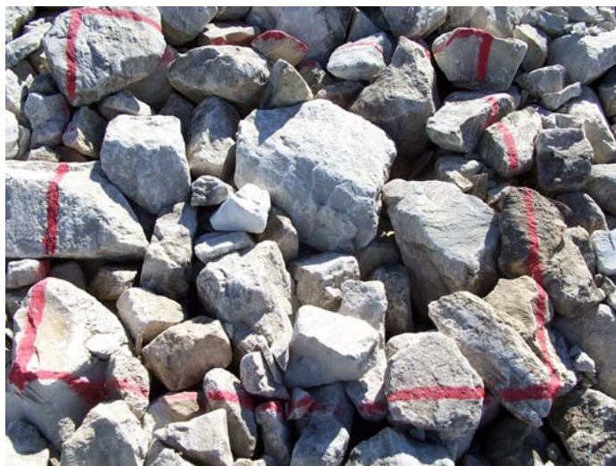
Photo 15. Cell cover rock test plot TP2; bottom of north side slope (2007 Inspection).
