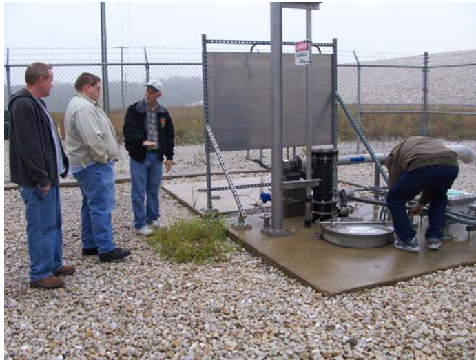
Photo 25. LCRS sump area.
