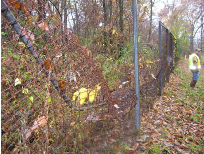
Photo 4. Damaged fence at the quarry.
