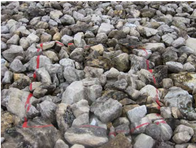
Photo 21. Cell cover rock test plot TP5; located on lower west side (2009 Inspection).
