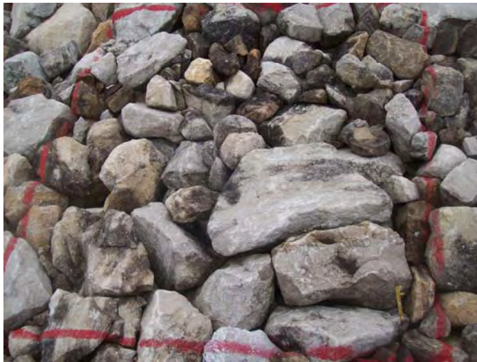
Photo 9. Cell cover rock test plot TP1; north edge of north facet (2009 Inspection).
