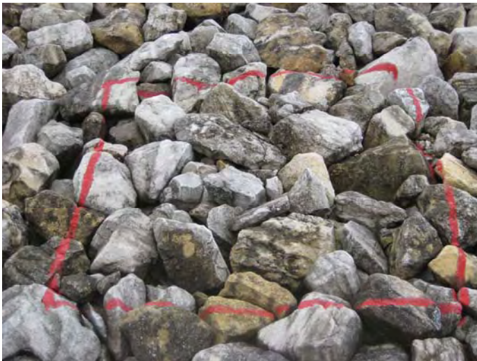
Photo 18. Cell cover rock test plot TP4; located on upper west side (2009 Inspection).
