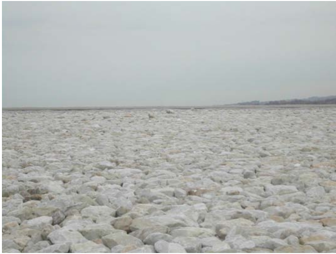
Photo 24. Rocks disturbed on top of cell.
