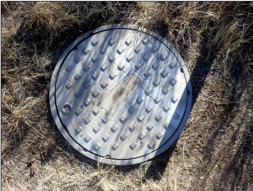
PL-3. Monitoring Well GJ84-04
