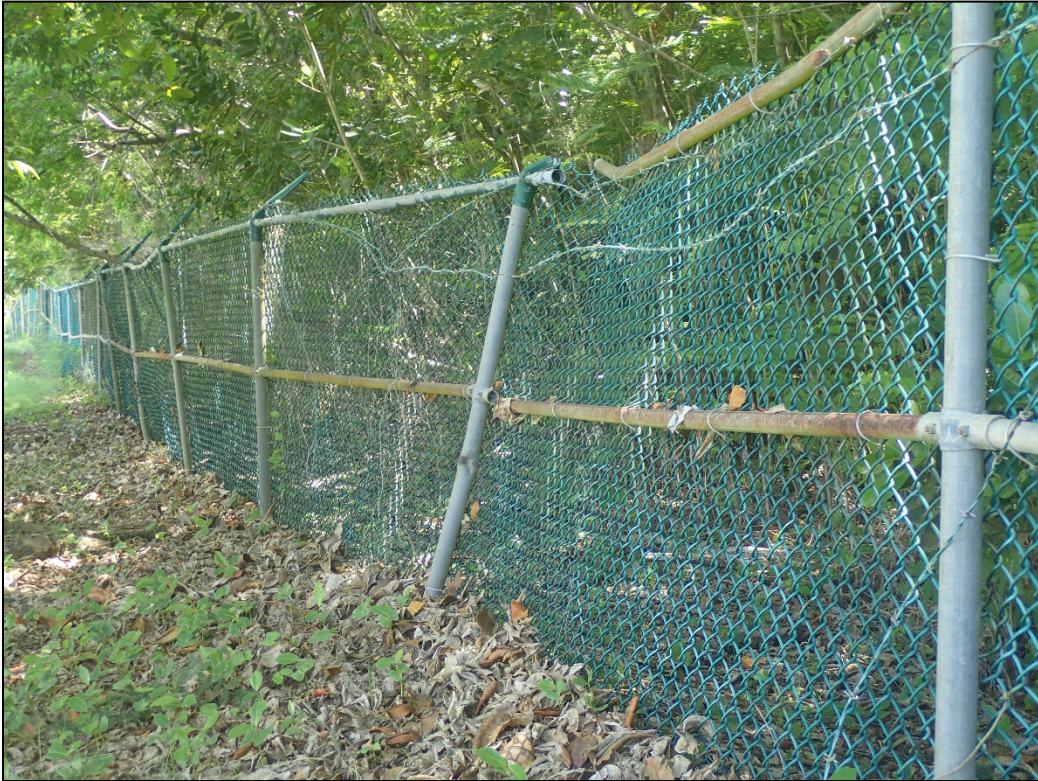
PL-6. Damaged Perimeter Fence
