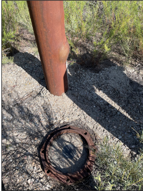
Photo 3. Example of Bollard Bulge
