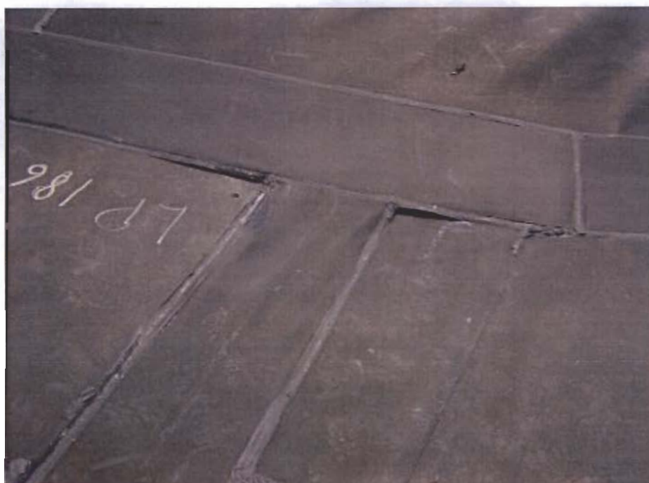
Photo 8: 2007 Seam Defect – Panel 186
