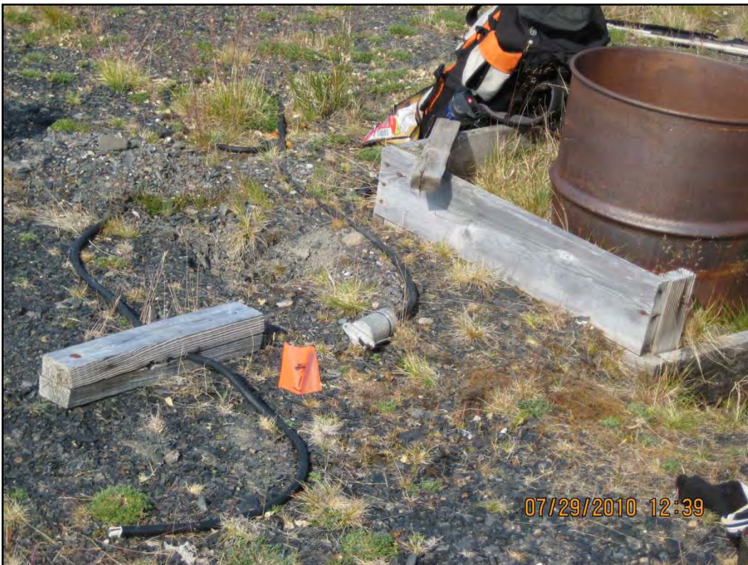
Photograph 18 – Thermistor cable installed through wood block near Test Hole Dog.
