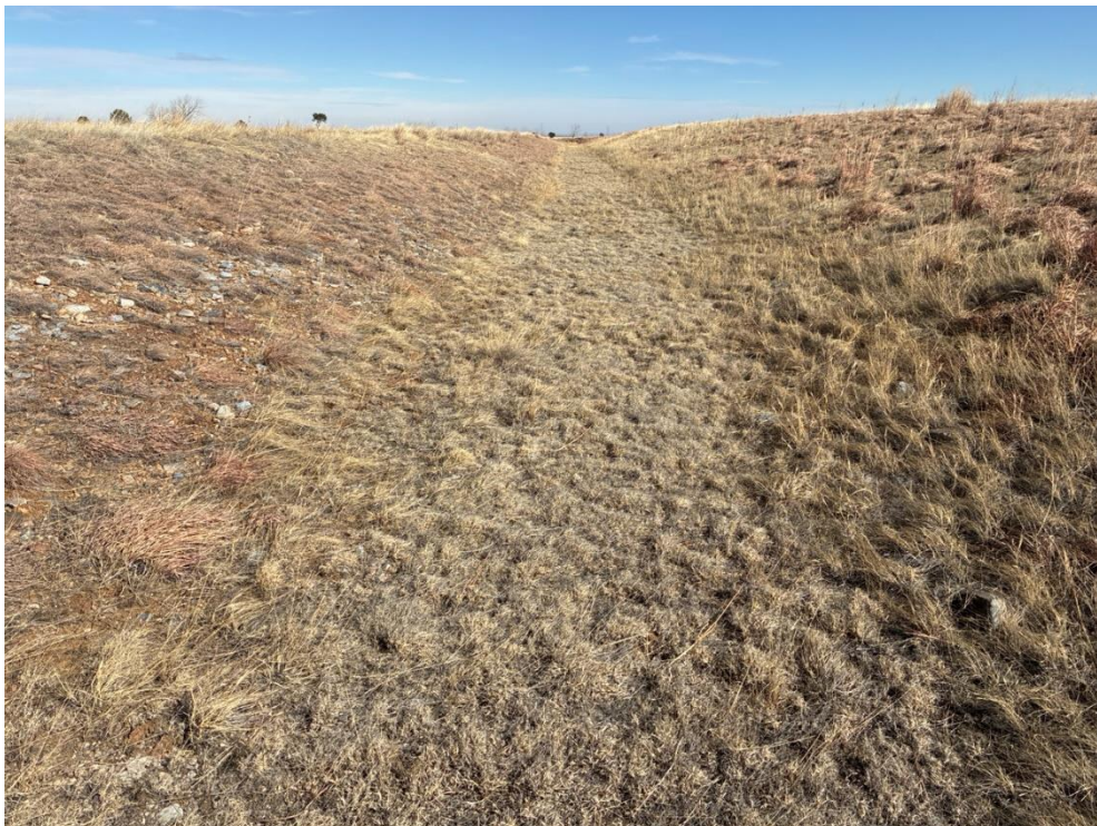
Figure 4. Looking Northeast at the Northern Vegetation-lined Perimeter Channel, Which Was in Good Condition.
