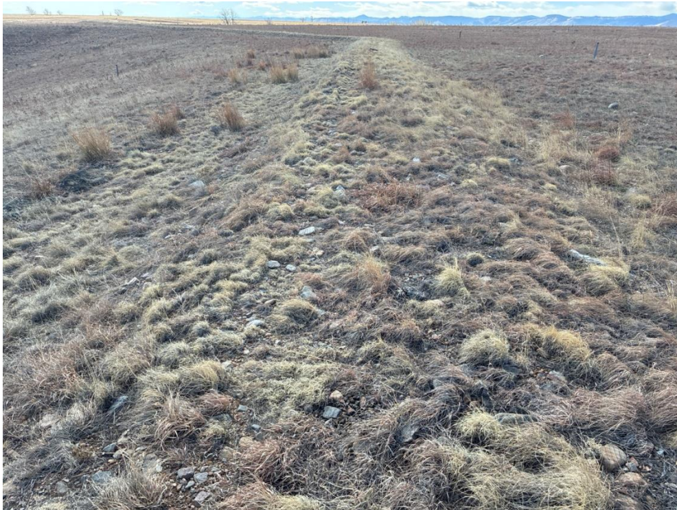
Figure 3. Looking South-Southeast at a Diversion Berm that Runs Along the Eastern Pediment, Which Was in Good Condition
