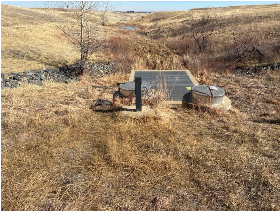
Figure 6. Looking East-Northeast at the Present Landfill Treatment System, Which Was Functioning Properly. Small amounts of bio-growth were removed from the North and South Manhole Outlet Pipes, treatment unit outlet pipe, and system outfall using a mechanical pipe cleaner as part of routine preventative maintenance.
