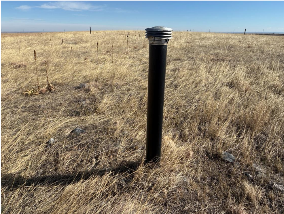
Figure 5. Looking Northeast at a Barometric Gas Vent on the Present Landfill Cover, Which Was in Good Condition.
