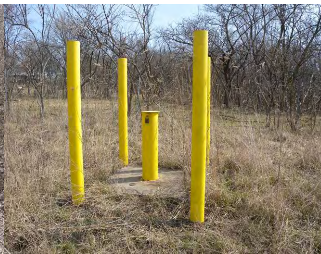
Figure 22. Parcel IB Well 0442, Locked, Labeled, and in Good Repair
