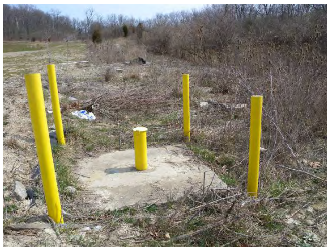
Figure 34. Parcel 9 MNA Well 0402, Locked, Labeled, and in Good Repair
