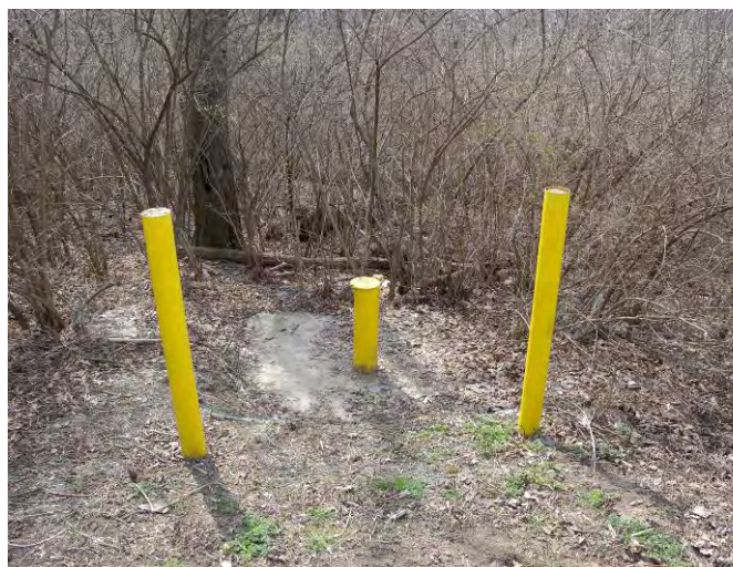
Figure 21. Phase IB Well 0411, Locked, Labeled, and in Good Repair
