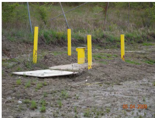
Figure 32. Parcel 9 MNA Well 0353, Locked, Labeled, and in Good Repair
