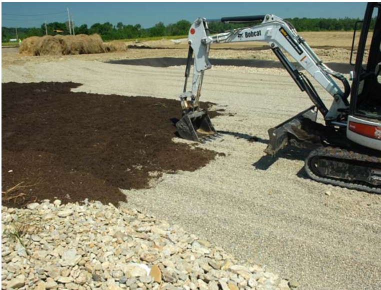
Fig. 1. The subsurface flow wetland gravel bed and mulch planting medium are being installed.
