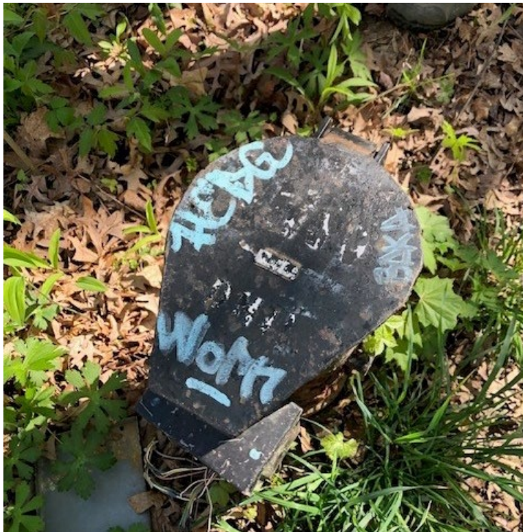
P13 – Monitoring Well DH11 at Red Gate Woods, Displaying Graffiti on Well Cap
